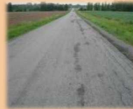
June 2008 REPAIRS NEEDED IN ORDER TO MAINTAIN PUBLIC SAFETY
