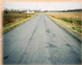
January 2006 FURTHER SNOW PLOW DAMAGE & WATER PUMPING AFTER 3RD WINTER 1/22/2016
