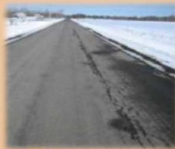
January 2007 DAMAGE CONTINUED NOW WATER IS PUMPING FROM SUBBASE
