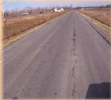
March 2004 FIBERMAT® TYPE A LONGITUDINAL CRACKS REAPPEARED AFTER 6 MONTHS 1/22/2016
