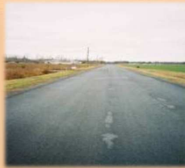
January 2005 FIBERMAT® TYPE A CRS-2p SNOW PLOW DAMAGE AFTER 2ND WINTER
